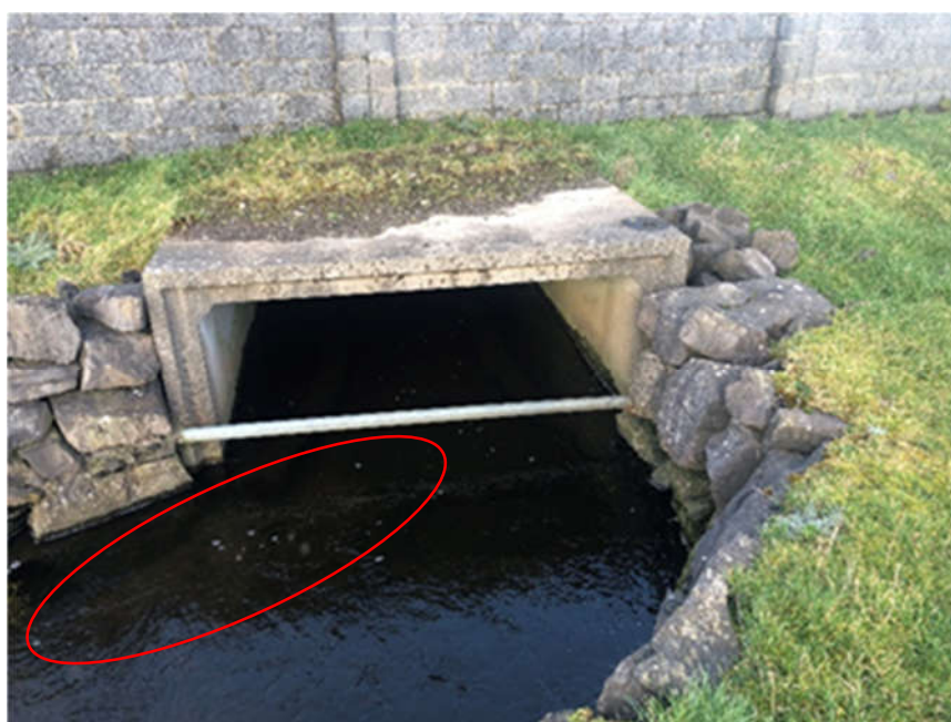
Plate 5-25 Silt build up at inlet to the culvert.
