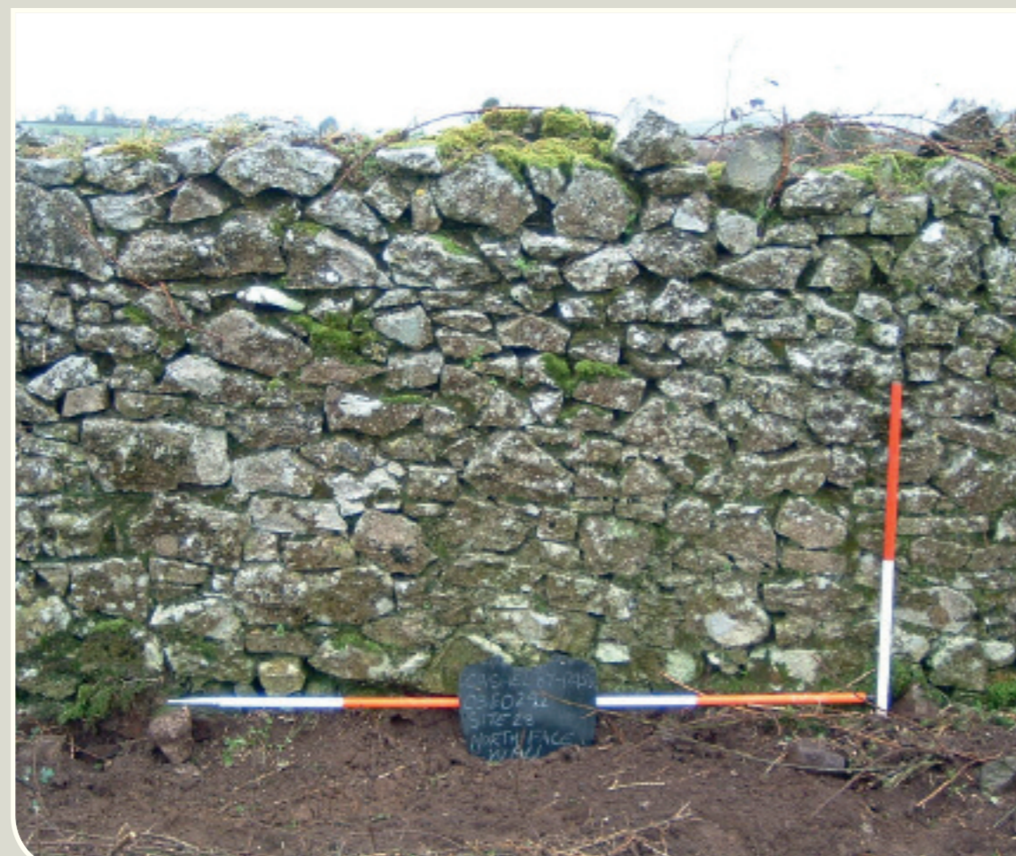
Townland wall built during Famine relief works at Rathordan . (Photo: Judith Carroll Network Archaeology)
