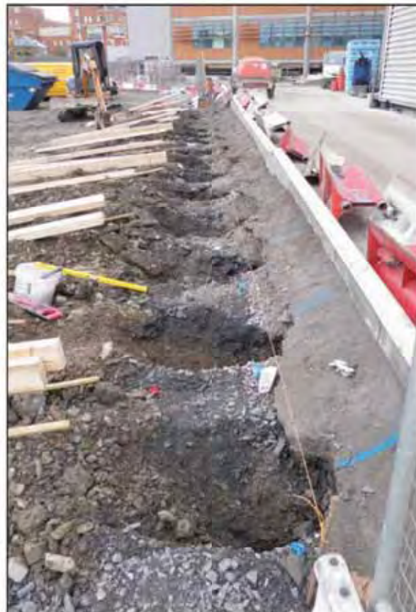
Plate 18. Monitoring of postholes associated with site hoarding along western boundary facing south.
