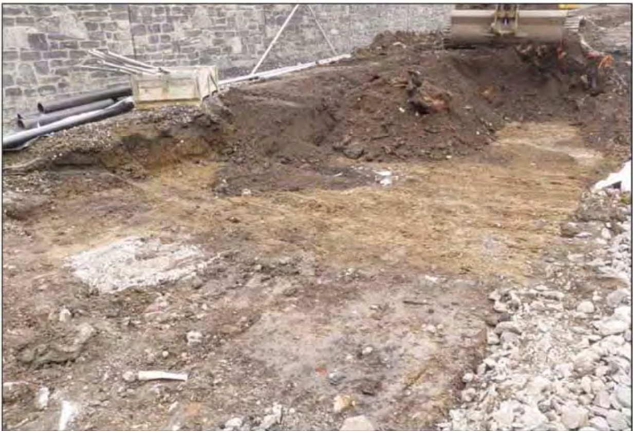
Plate 22. Monitoring of overburden removal along eastern side of the site facing south.
