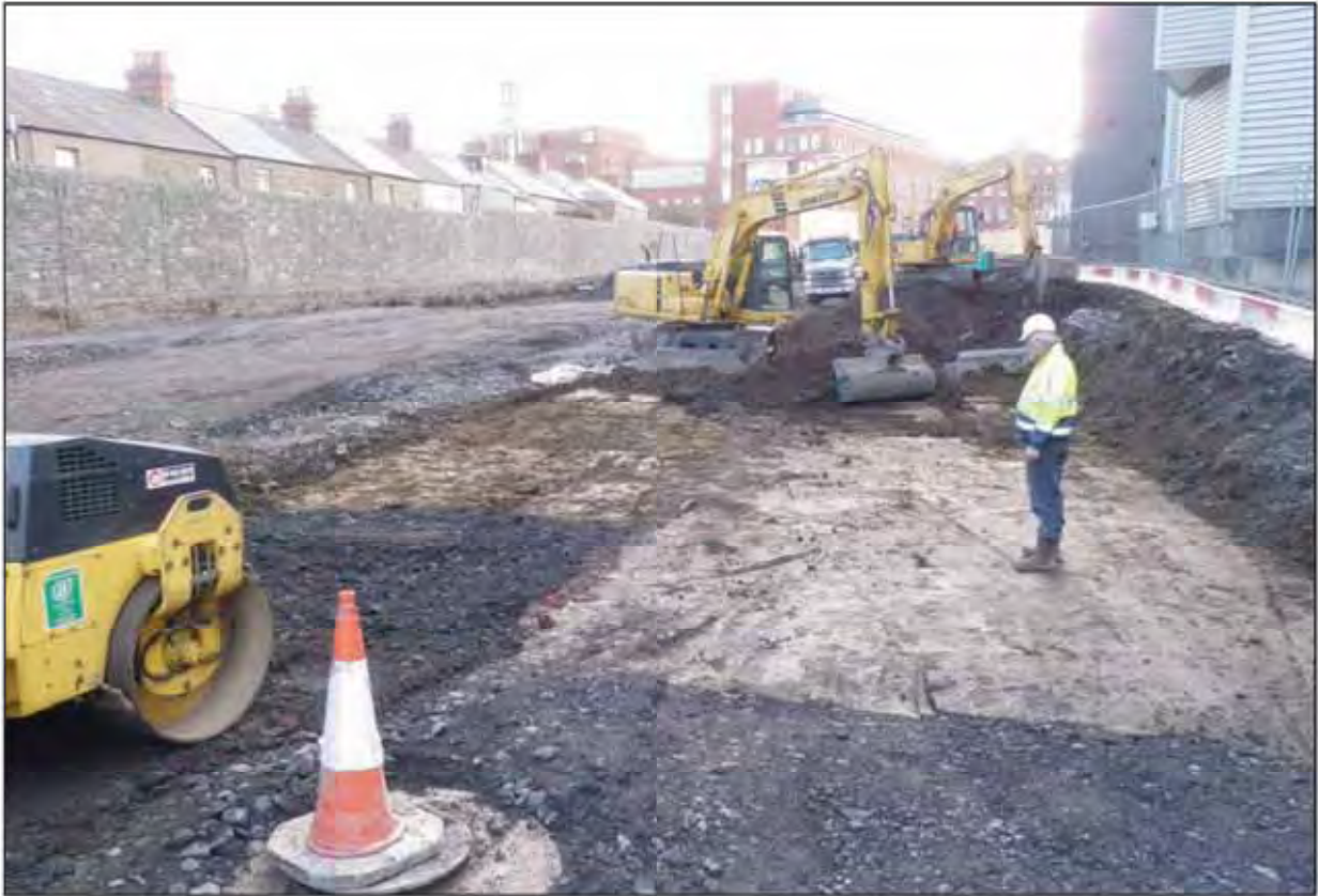
Plate 23. Monitoring of overburden removal along western side of the site facing south.
