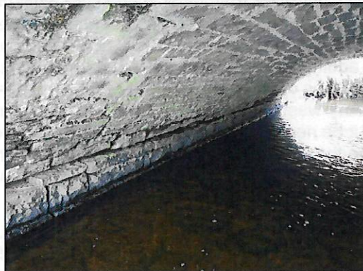
Plate 3. Stonework requiring repointing at base of arch [Source: Atkins R.E.; 26/10/2018].
