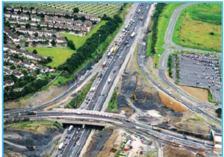
▶ M50 Upgrade Contract 1 (N4 Interchange at Palmerstown to North of N81 Tallaght)
