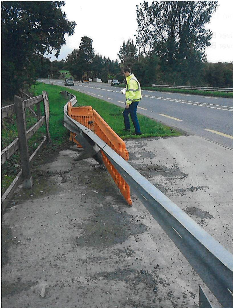
Plate 2. Damaged Guardrail on Bridge
