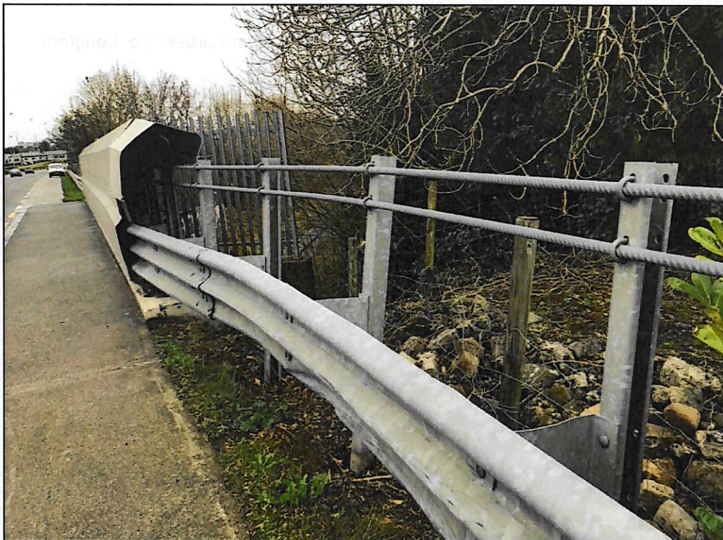
Plate 1. Damage to transition area
