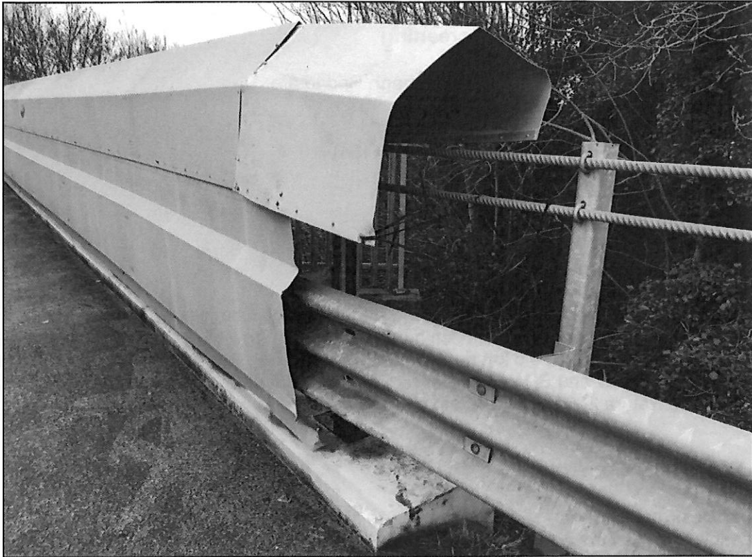
Plate 2. Damage to parapet
