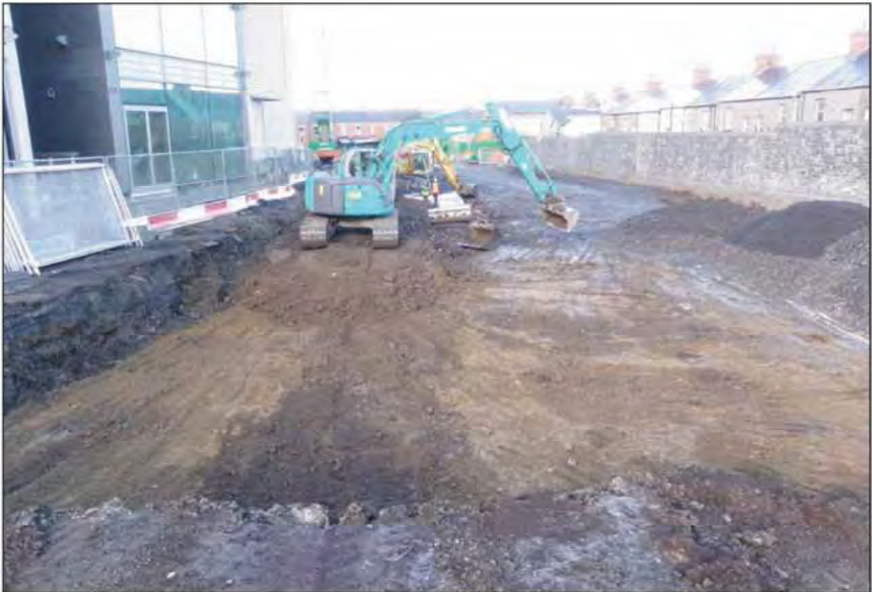
Plate 26. Outline of sewerage main evident along western side of the site facing north.
