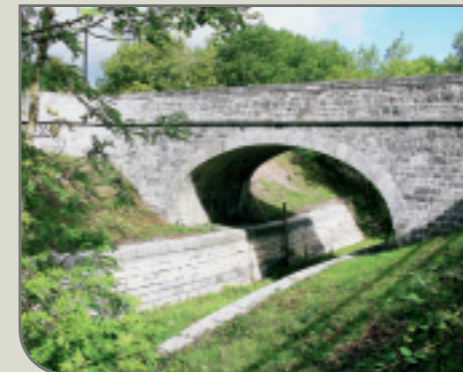
An early 19th-century road bridge on the Connaught extension of the Grand Canal. (Photo: Studio Lab)
