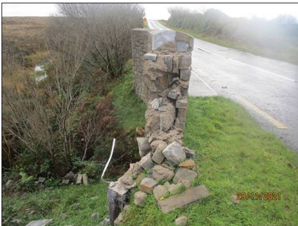
Plate 1 Damage to Bridge parapet.
