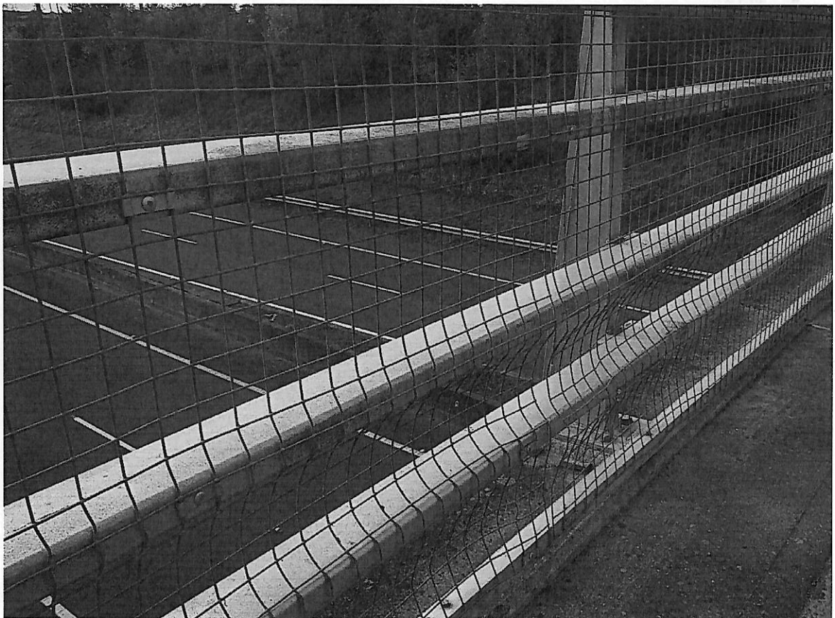
Plate 1. Damaged mesh panel on parapet
