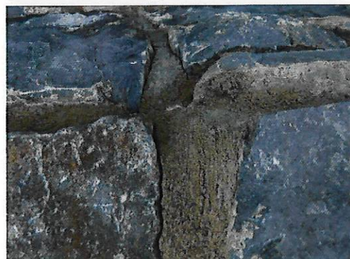
Plate 2. Parapet wall requiring masonry repair.
