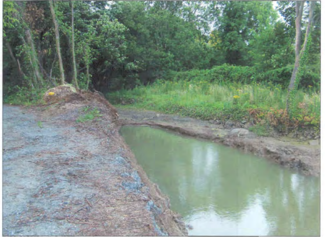
Plate 6 View SE of dredged Carrickmines River watercourse (note rock armour along far bank)
