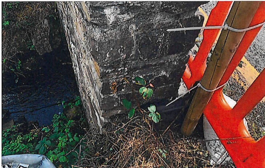
Plate 3. The wall structure is coming away from the kerb.
