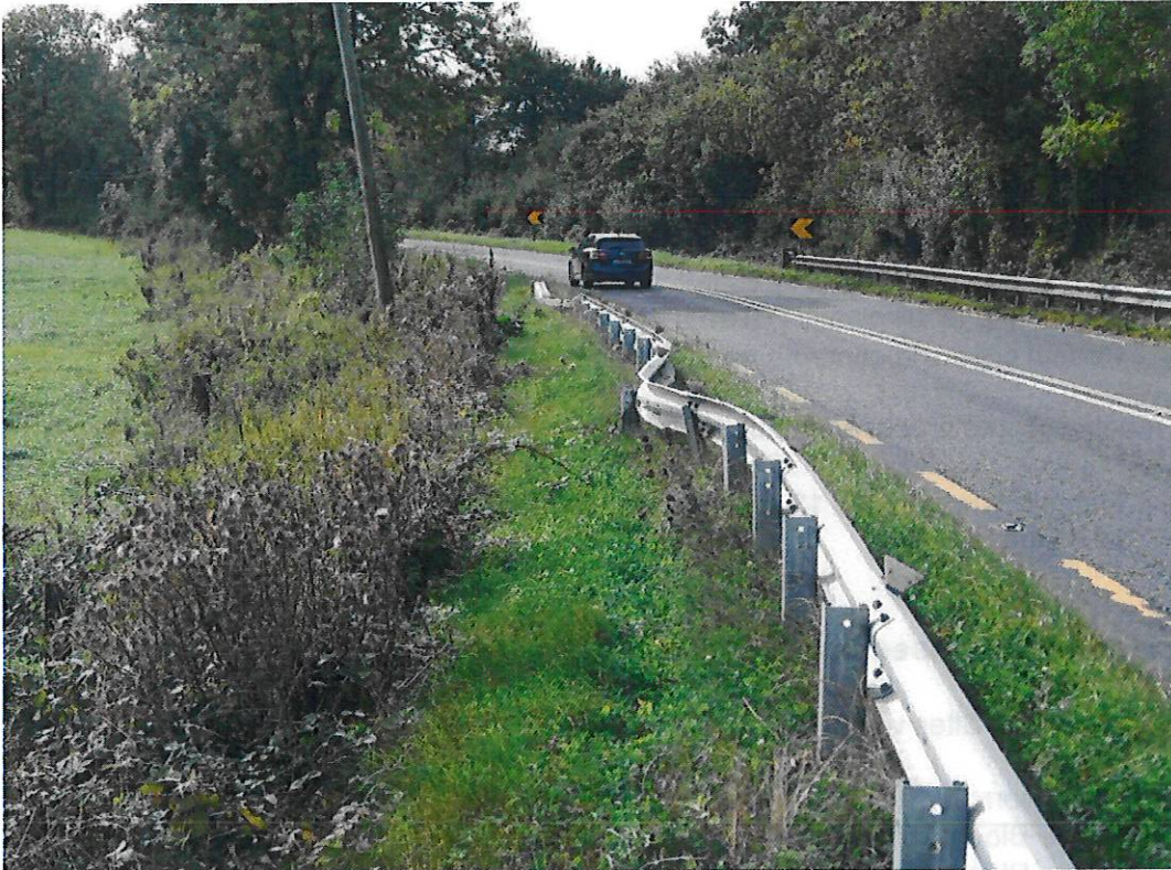
Plate 2. Damaged Crash Barrier
