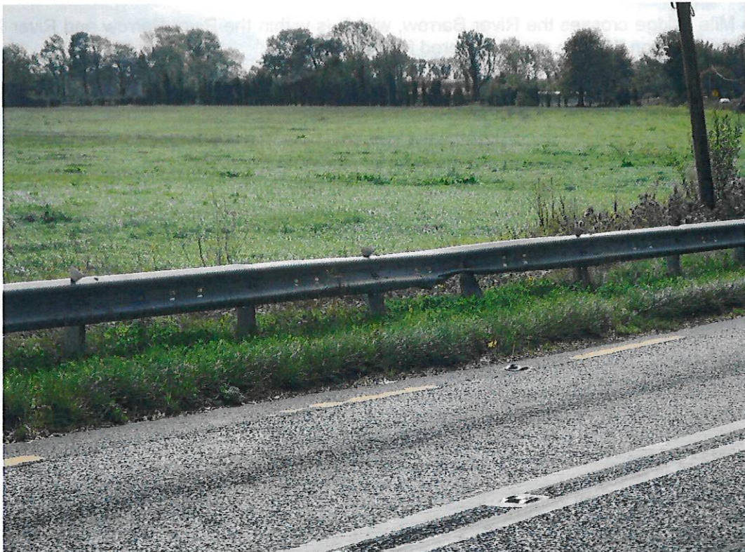
Plate 3. Damaged Crash Barrier
