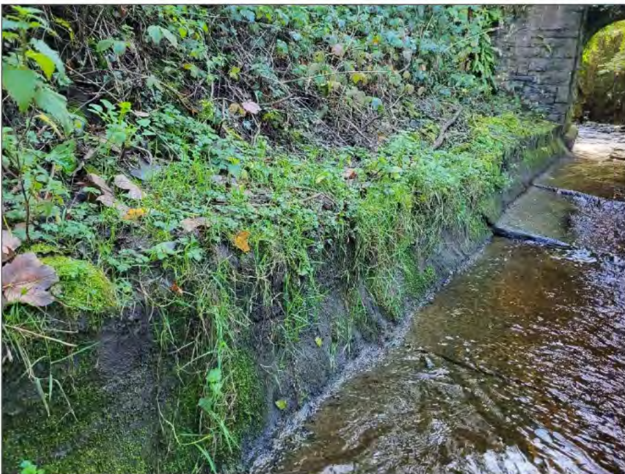
Plate 1-8 Upstream of culvert eastern bank, apron damage visible.
