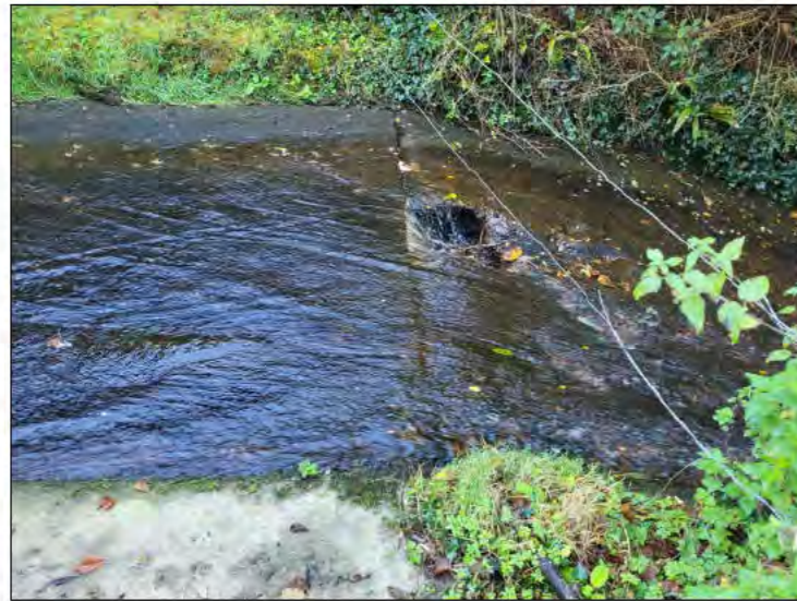
4. VOIDS AND CRACKS TO DOWNSTREAM APRON No. 1
