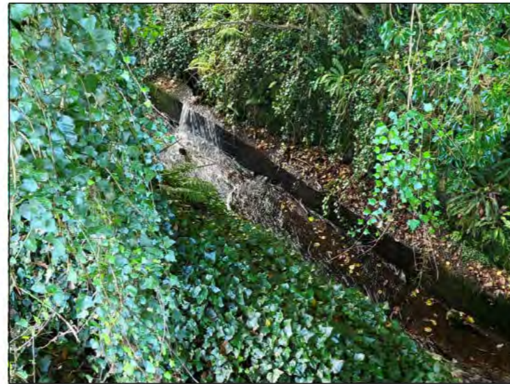
5. VOIDS AND CRACKS TO DOWNSTREAM APRON No. 2
