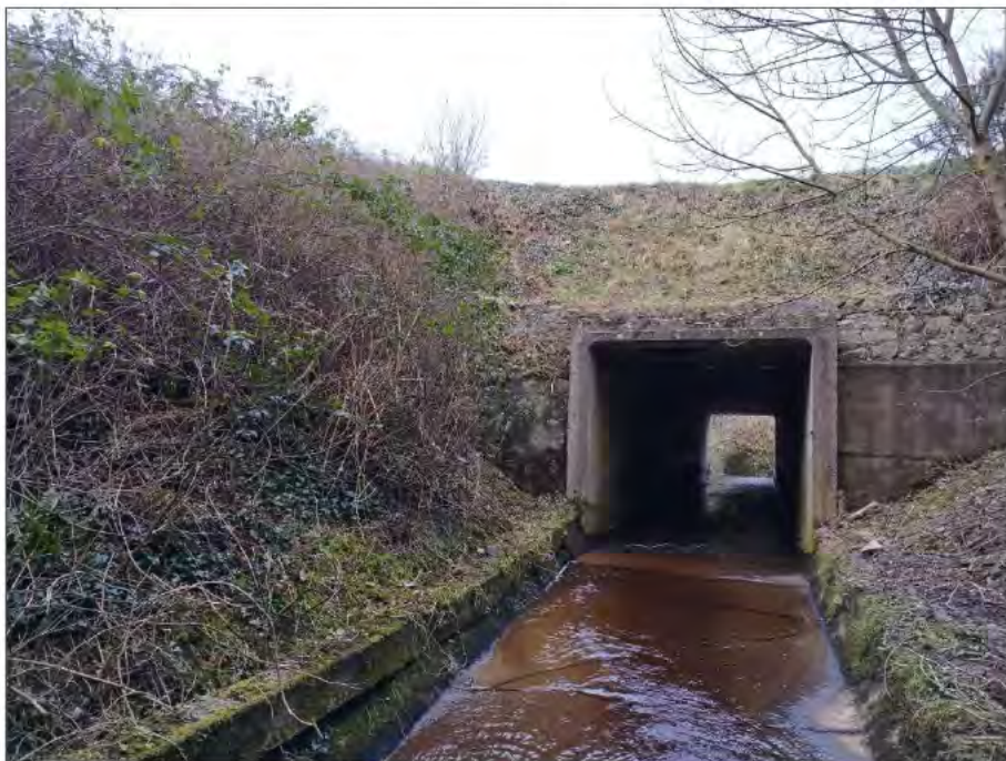
Plate 4-1 View of Knockbrack Culvert looking downstream, scrub visible on the western bank.
