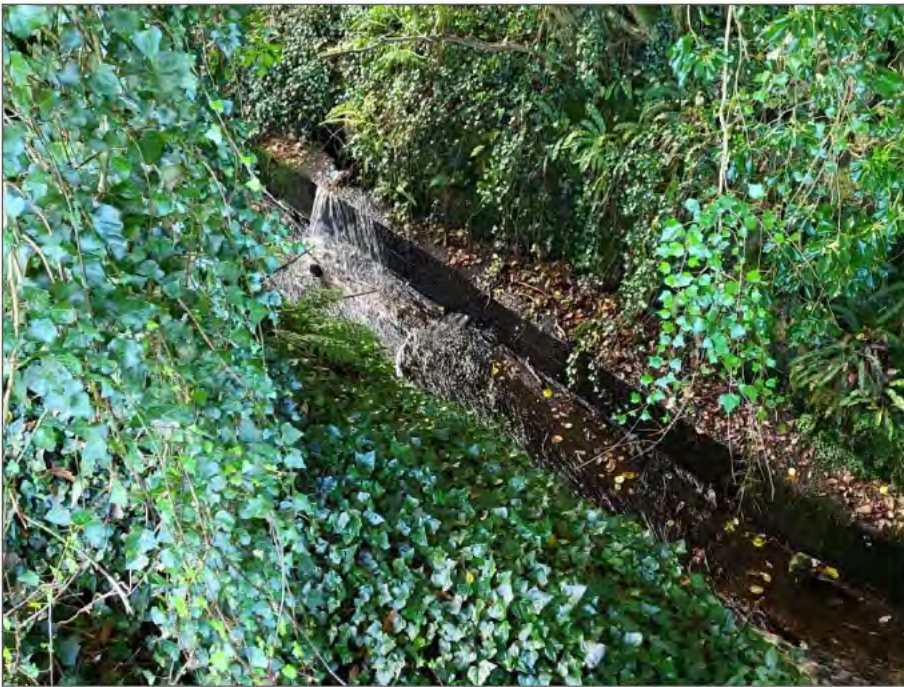
Plate 1-4 Defects to apron downstream of culvert.
