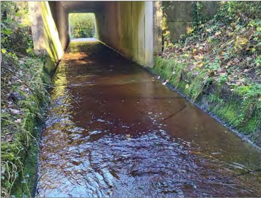
Plate 1-7 Upstream of culvert looking downstream, apron damage visible.
