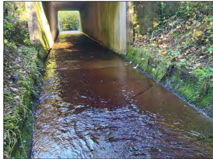
8. CRACKING TO UPSTREAM APRON
