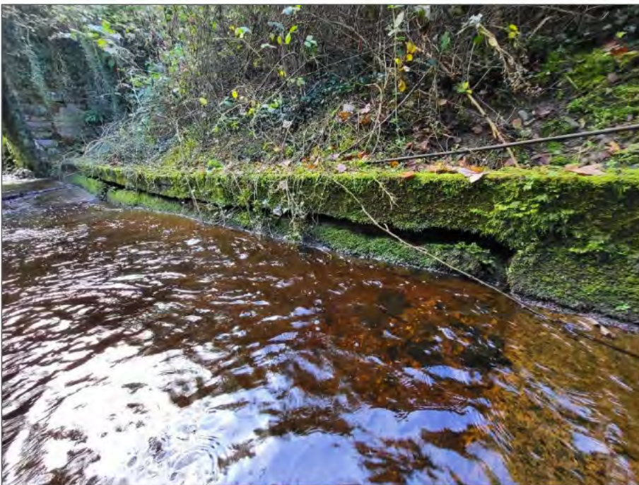
Plate 1-6 Damage to existing plinth upstream of culvert, western bank.
