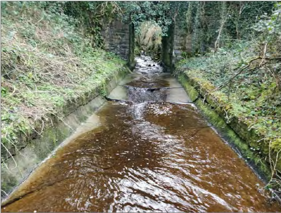
Plate 1-5 View of apron damage looking upstream of culvert looking towards old railway bridge.
