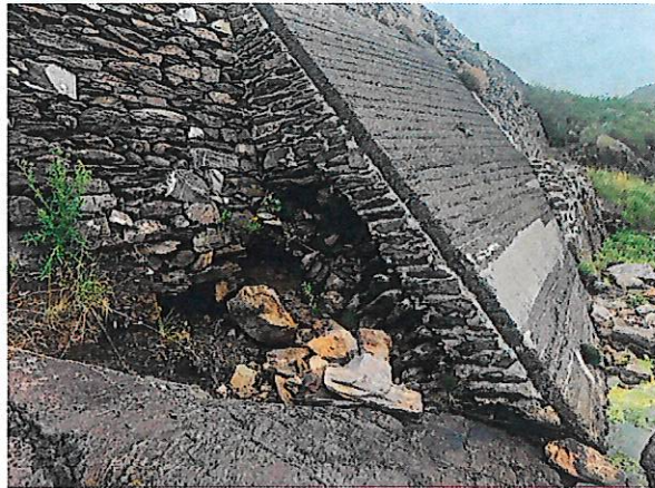
Plate 2. Close-up of erosion of retaining wall and buttress.
