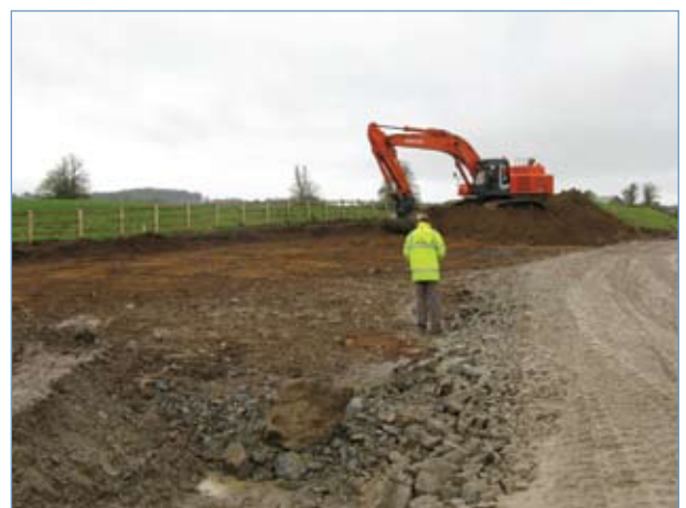
Excavation of Topsoil on the N7 Castletown to Nenagh Scheme (Photograph courtesy of KCC NRDO)
