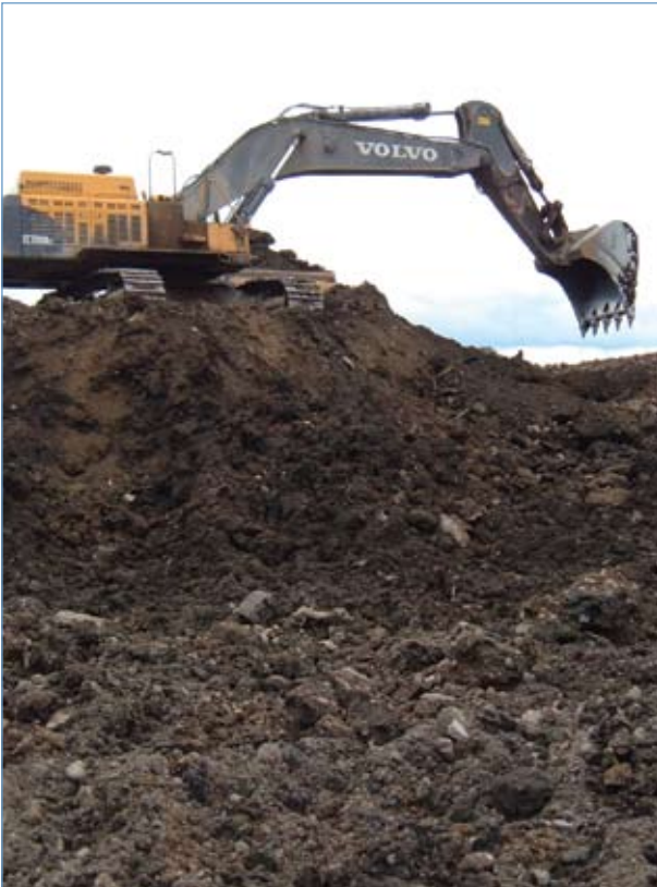
Bulk Excavation of Inert Construction and Demolition Waste (Photograph courtesy of Roadbridge Ltd).JPG
