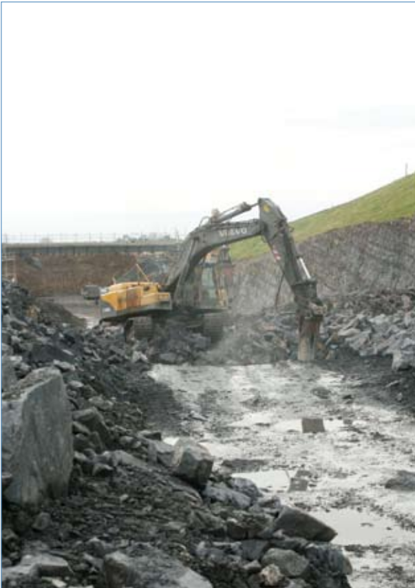
Rock Breaking Activity on the M8N8 Cashel to Cullahill Scheme (Photograph courtesy of SRB Civil Engineering Ltd (a joint venture between Roadbridge Ltd and John Sisk & Son Ltd))
