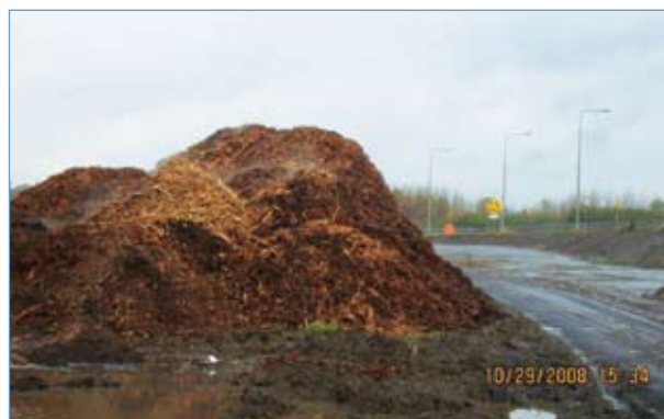
Mulching of Existing Vegetation on the M7M8 Motorway Scheme (Photograph courtesy of the Office of the NRA's Representative)
