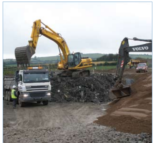
Excavation and Removal of Municipal Solid Waste to Landfill (Photograph courtesy of Roadbridge Ltd)
