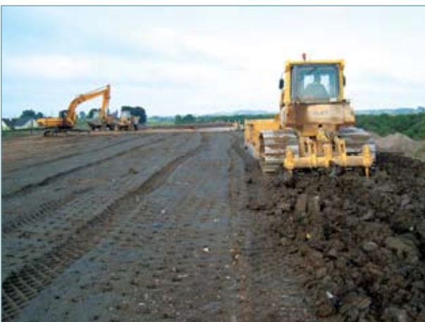
Reworking of Inert Construction and Demolition Waste to Suitable Material following Screening (Photograph courtesy of Roadbridge Ltd).JPG
