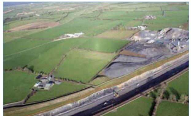
Rock Processing on the M8N8 Cashel to Cullahill Scheme (Photograph courtesy of SRB Civil Engineering Ltd (a joint venture between Roadbridge Ltd and John Sisk & Son Ltd))
