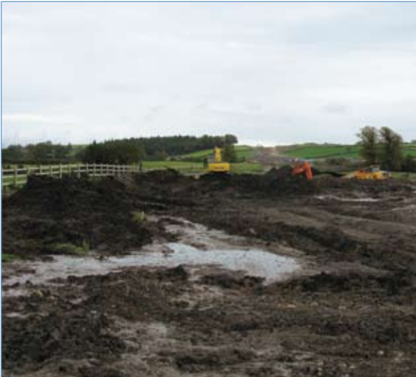
Excavation of Peaty Material on the N7 Castletown to Nenagh Scheme (Photograph courtesy of KCC NRDO).JPG
