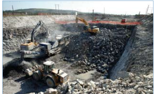
Rock Crushing on the M8N8 Cashel to Cullahill Scheme (Photograph courtesy of SRB Civil Engineering Ltd (a joint venture between Roadbridge Ltd and John Sisk & Son Ltd))
