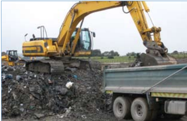
Excavation and Removal of Municipal Solid Waste to Landfill (Photograph courtesy of Roadbridge Ltd)
