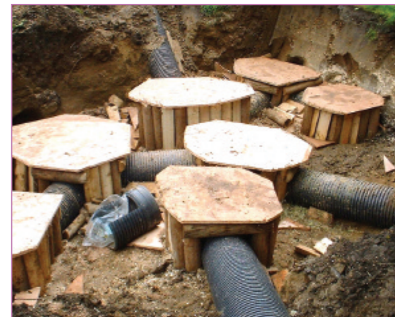
An example of an artificial sett under construction, with pipe tunnels and eight chambers.
