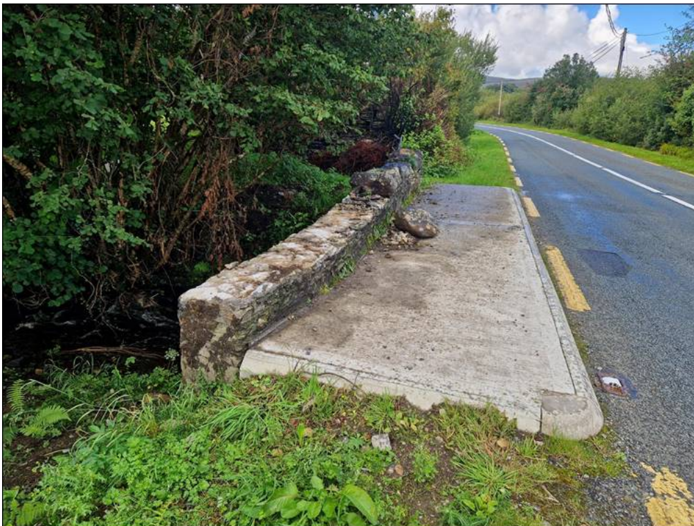
Figure 2: Damaged section of the coping to be reinstated at Carrowvagh Bridge (MO-N59-053.50).
