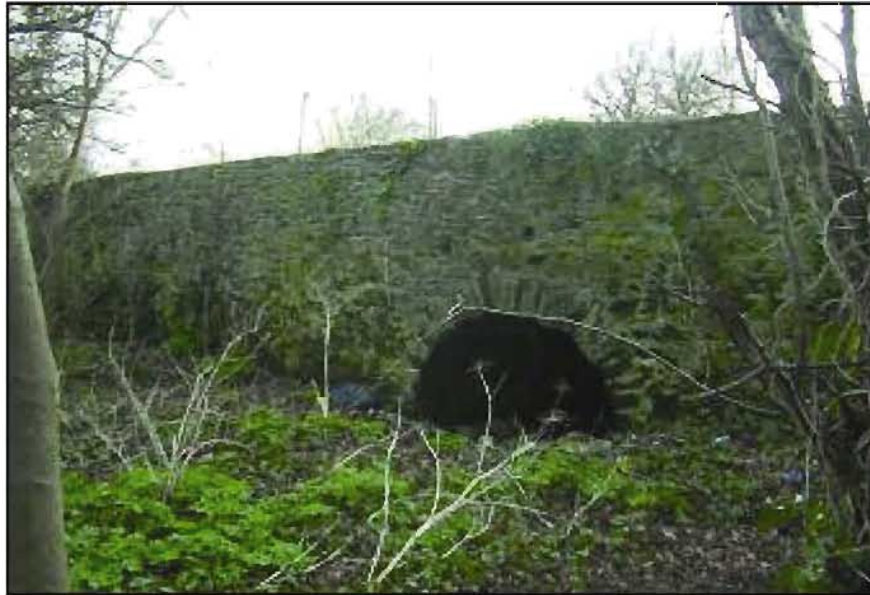
Plate 9 - Photograph of visible arch/culvert within existing western wall of Lissenhall Bridge (HC#11), facing northeast.
