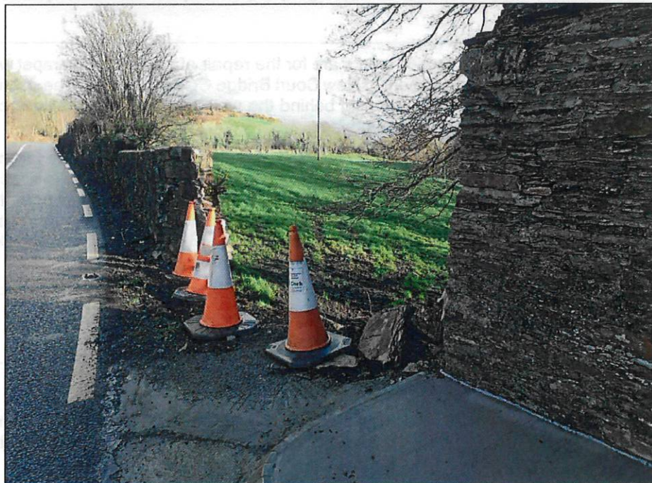
Plate 2. Damaged parapet wall [Source: Atkins R.E.].
