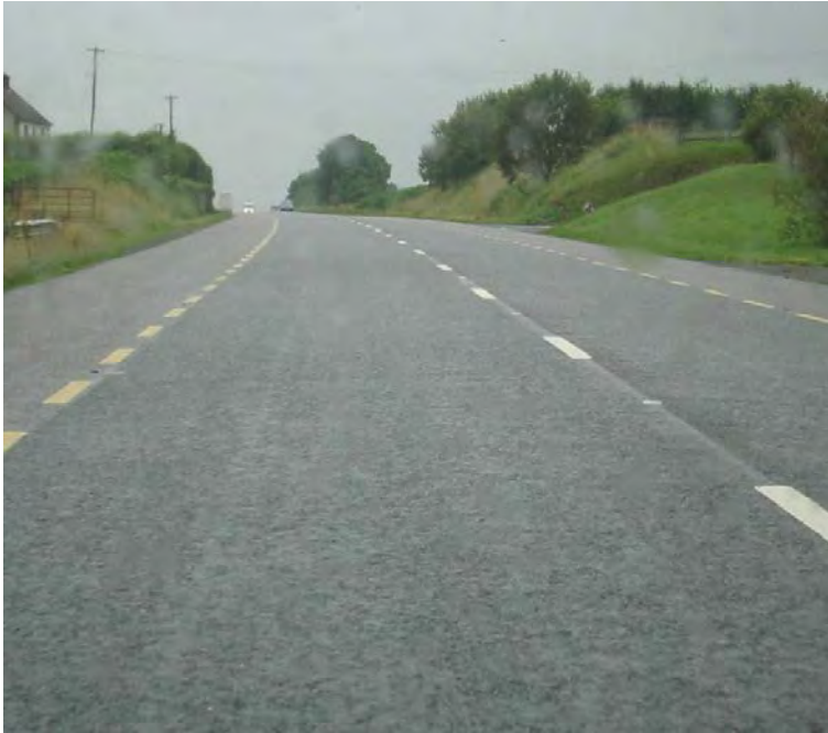
Before road safety remedial measure implemented
