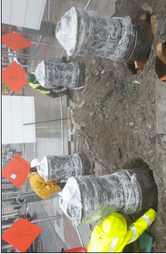
Plate 1: O'Connell St. Upper; Parnell National Monument; removal of fill material from base of bollards
