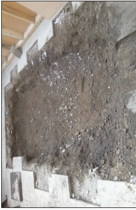
Plate 4: Grafton St.; Molly Malone statue original location; view of area following removal of foundation.
