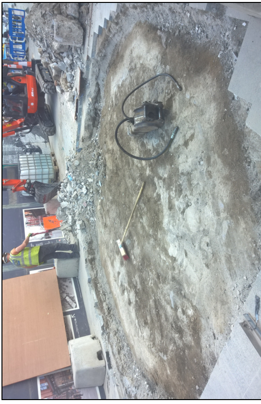
Plate 10: O'Connell St. Upper; Fr. Mathew statue; view of area following removal of foundation.
