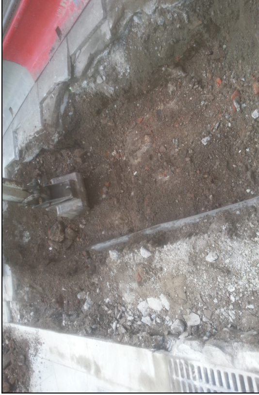
Plate 5: St. Andrew St.; Molly Malone statue new location; new foundation trench under excavation.
