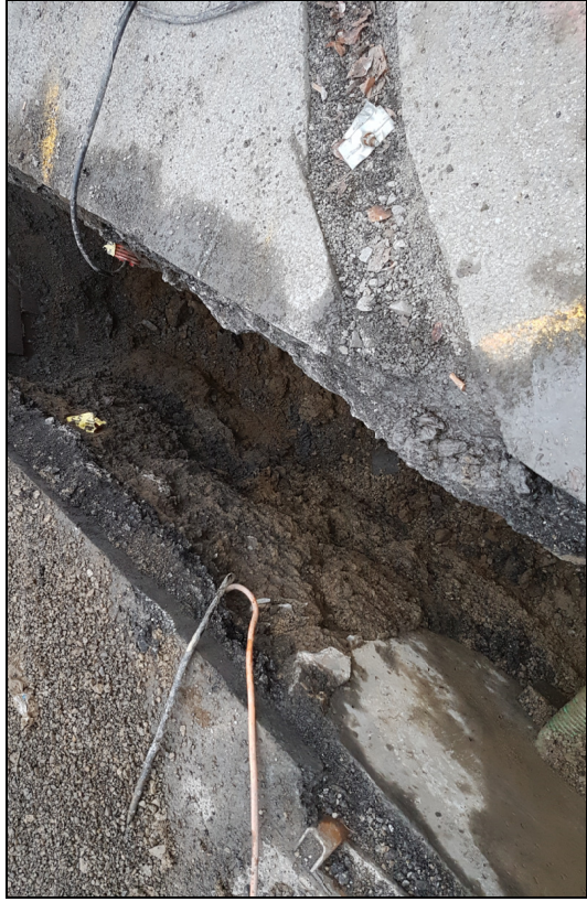
Plate 11: St. Stephen's Green; Lady Grattan statue new location; view of watermain trench
