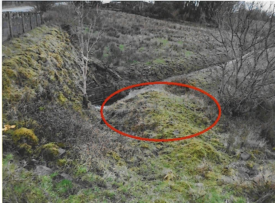
Plate 4. Mound of material to be regraded to a 45 degree slope (circled in red).
