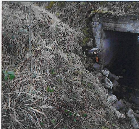
Plate 2. Wall collapse on the downstream side of Coolloughra Bridge.
