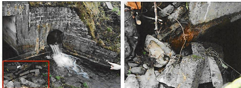
Plate 5. Debris within the channel (collapsed wingwall)
