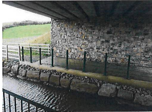
Plate 3. Revetments requiring cleaning and sweeping [Source: Atkins R.E.; 10/2018]
