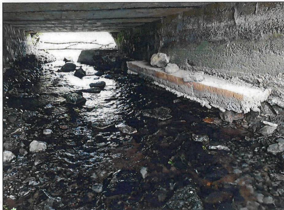
Plate 2. Undermining of left abutment.
