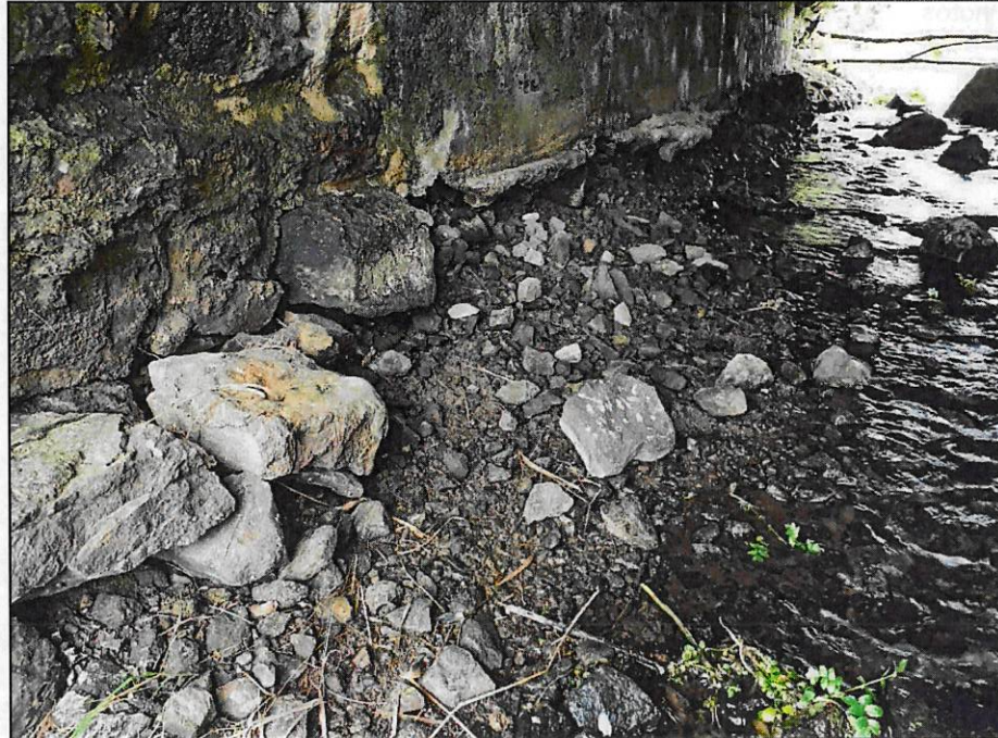
Plate 3. Undermining of right abutment.
